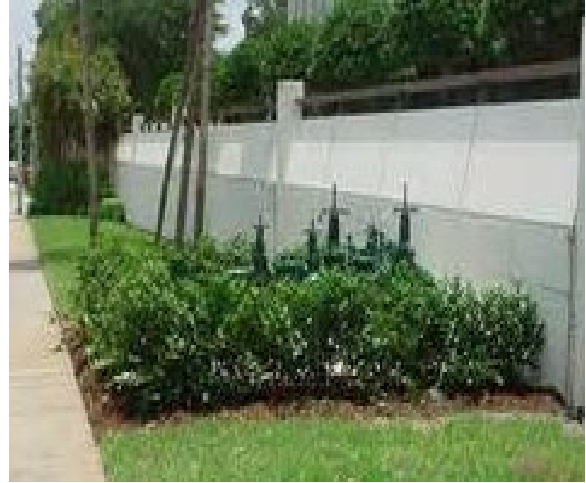
Bushes Screening Backflow Prevention Assembly
