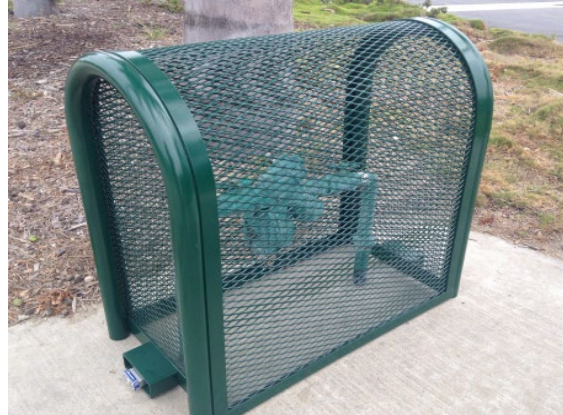
Residential Backflow Prevention Assembly with Locked Enclosure
