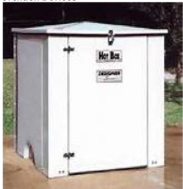
Freeze-protected Fiberglass Enclosure Over Backflow Prevention Assembly
