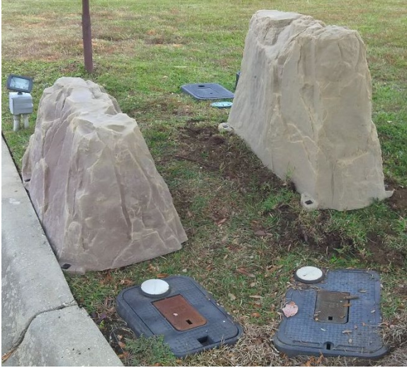
Faux Rocks Covering Backflow Prevention Assemblies
